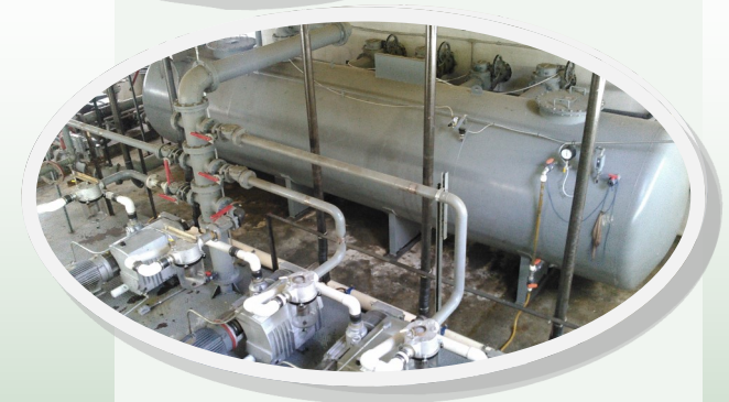
Wastewater Collections System Meadow Creek Vacuum Station #2 Meadow Creek Church Rd Locust NC
