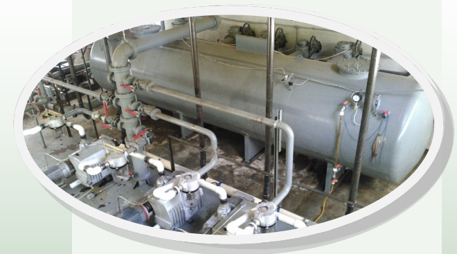
Wastewater Collections System Meadow Creek Vacuum Station #2 Meadow Creek Church Rd Locust NC
