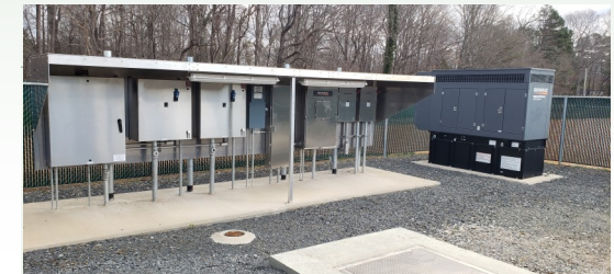
Wastewater Collections System Town Center North Lift Station #11 Kerri Dawn Ln Locust NC
