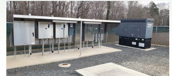
Wastewater Collections System Town Center North Lift Station #11 Kerri Dawn Ln Locust NC
